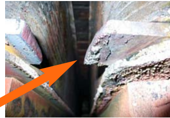
Rotor pole joint failure
