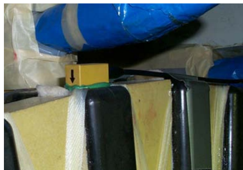
FOA-100™ being installed on an air-cooled unit at the Astoria power plant
