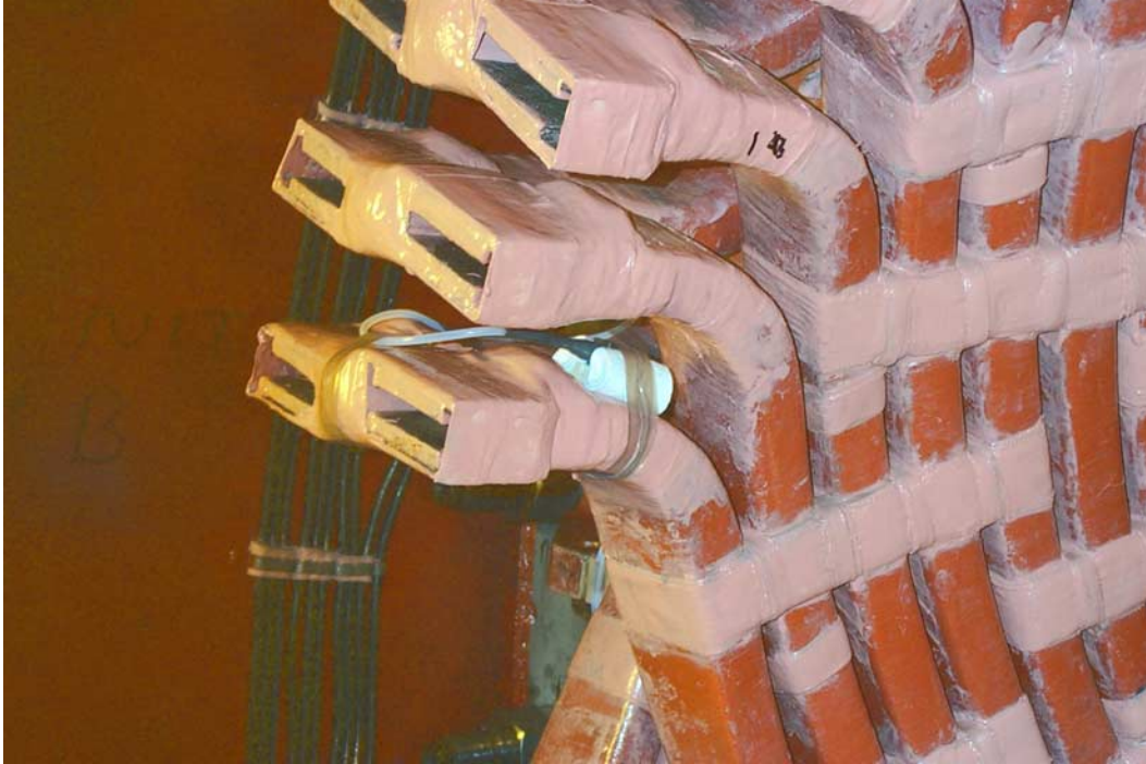
FIGURE 2 – Sensor head and optical cable temporarily secured to the end-winding
