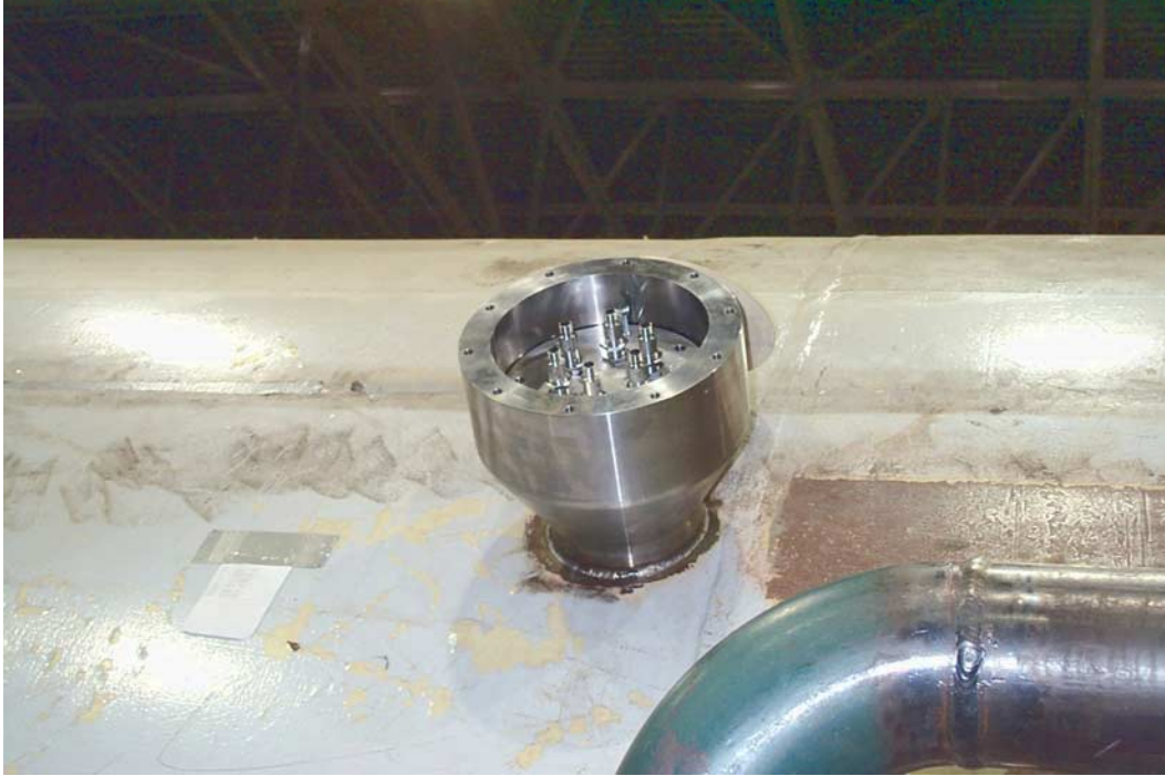
FIGURE 3 – Sealed flange welded on the generator casing with feedthrough connectors ready to connect. When external instrumentation is not connected, a sealed plate is placed over the opening to provide additional security
