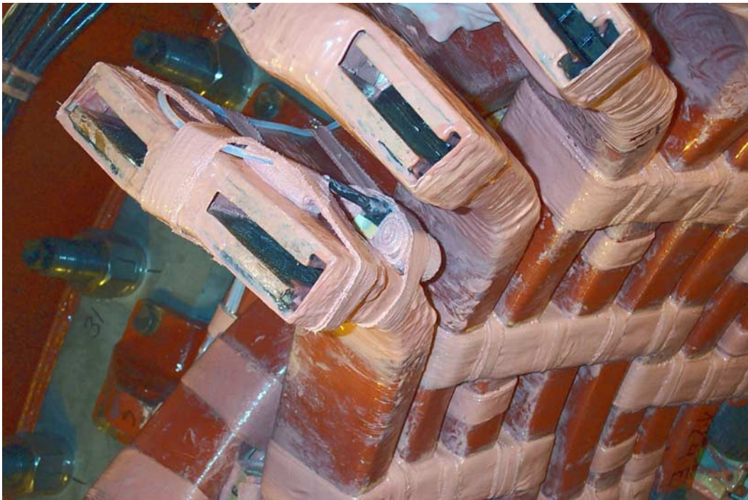
FIGURE 4 – Final installation of the sensor head and optical cable with same impregnated material used to brace the end-windings
