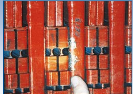
Paint flaking on end-windings caused by vibration contacts against laminations.
