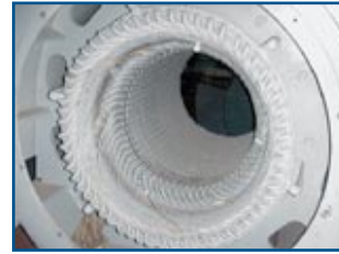
Large Electric Motors
