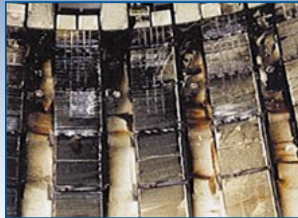
Deposit of oil mist on end-windings and stator core at extremities contributing to bar vibration.
