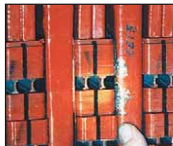
Paint flaking on end-windings caused by vibration contacts against laminations.
