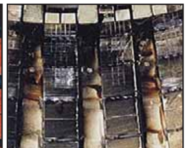
Deposit of oil mist on end-windings and stator core at extremities contributing to bar vibration.
