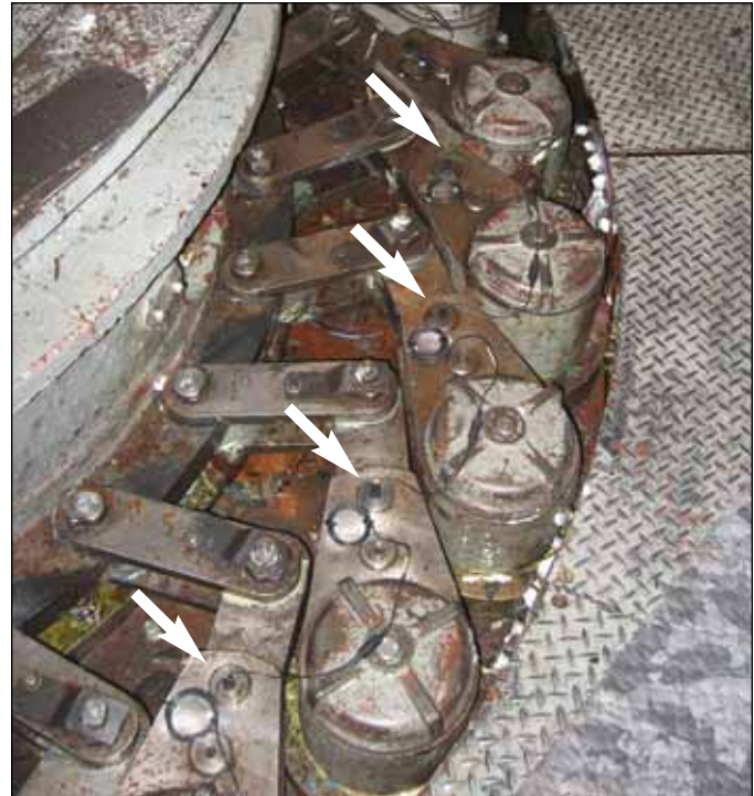
VibroSystM's Broken Shear Pin Detector installed on hydroelectric machine.
